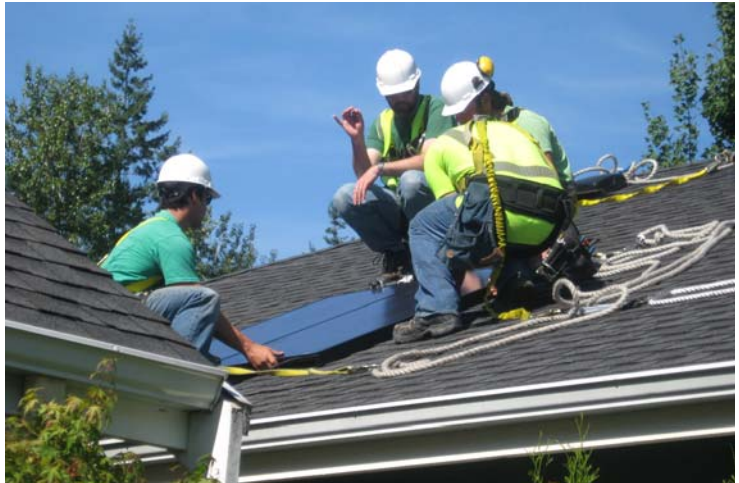
PHOTO CREDIT: PUGET SOUND SOLAR
